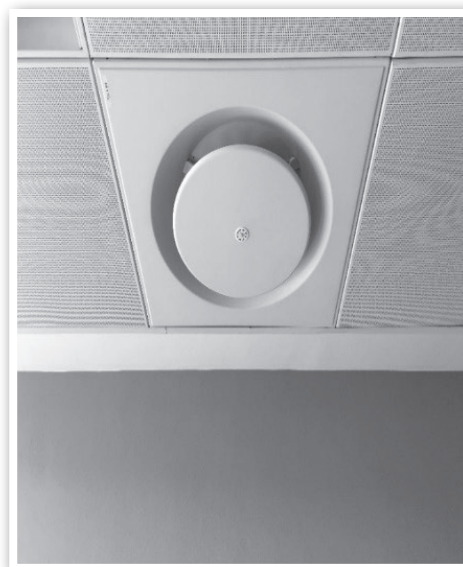
New energy-efficient diffusors installed on Floor 1
