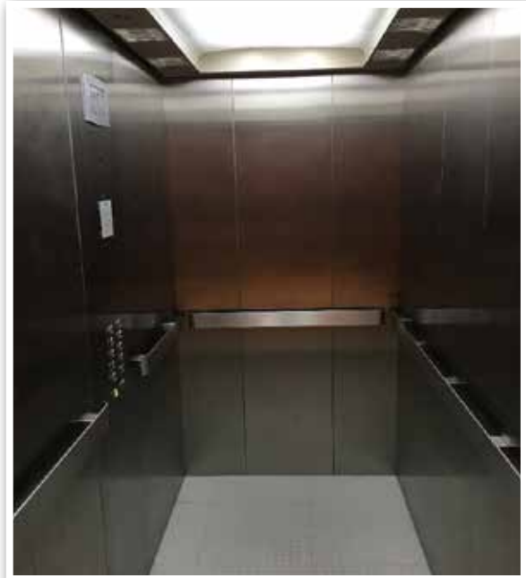
New Goods Elevator
