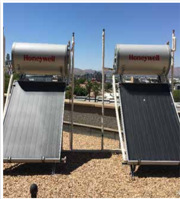
Solar Geysers for Cafeteria
